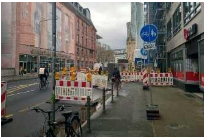
Fig. 6. Traffic signalization (R. Germany)
