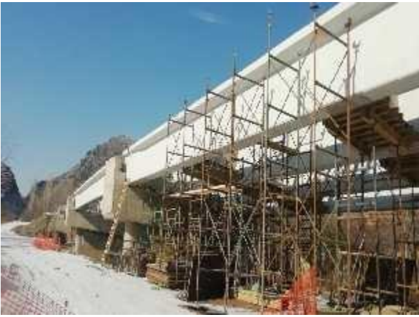
Fig. 2. Construction site of road infrastructure facility, express road Prilep-Gradsko, R. North Macedonia
