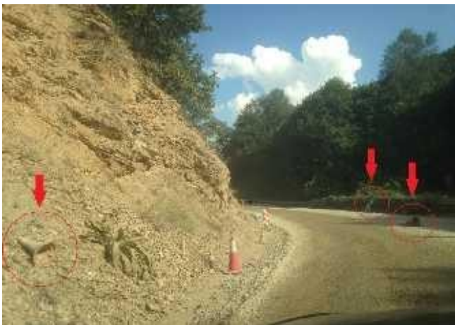
Fig. 7. Reckless operation of a construction site
