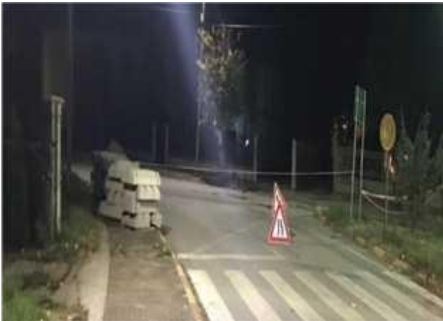
Fig. 3. Improper signage in front of the construction site
