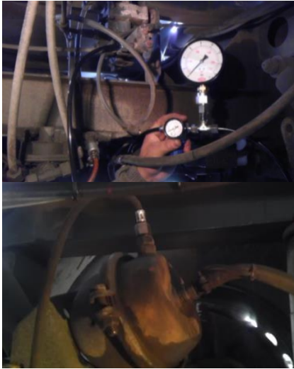
Fig. 6 Position of the pressure regulator in the cushion as well as the connection point on the brake cylinder for pressure measurement.
