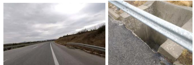
Fig. 2. Entrance head from pipeline omission, \text{km}15 + 830 (west lane)
